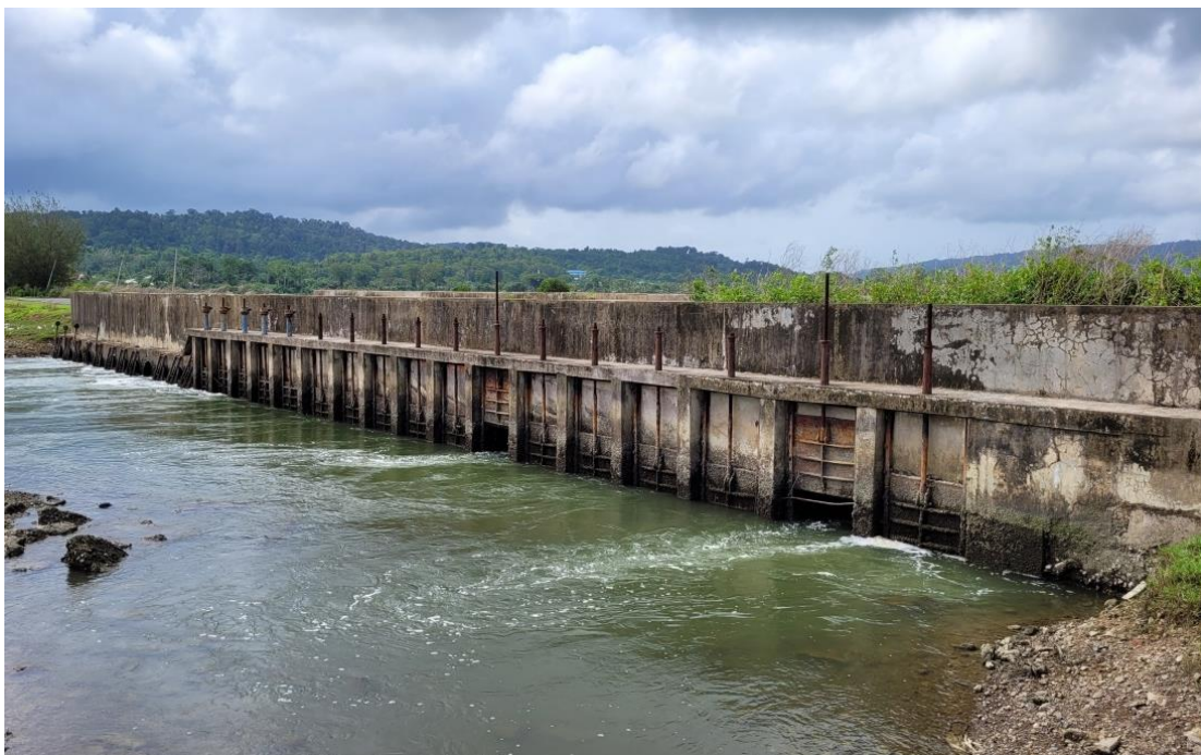
Photograph 12. The sluice gate near Stewartgunj village was severely damaged during the 2004 tsunami. Although it was repaired, the extensive damage makes full restoration became difficult.
